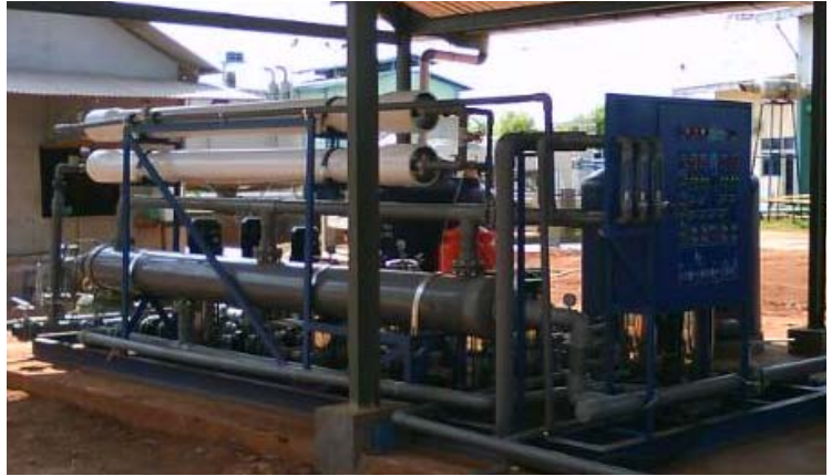
Non-modular Ultrafiltration has been used as pretreatment for LPRO on industrial water treatment unit
