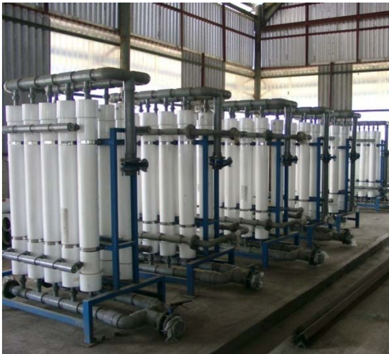
Modular Ultrafiltration Plant Needs Complex Piping System and Requires More Instruments
